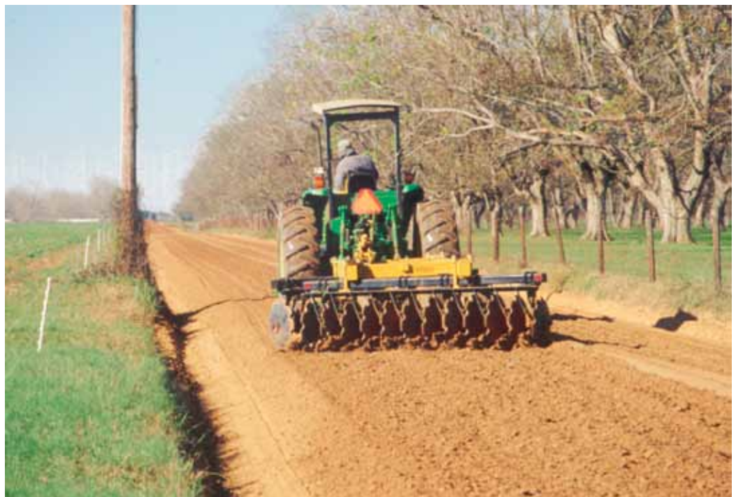
Stabilizer products being mixed into road soil before compaction in Baldwin County, Alabama.
