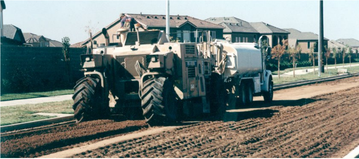
Mixing of 12-inch layer of subgrade soil using pulverizer and water truck with EMC SQUARED treated water.
