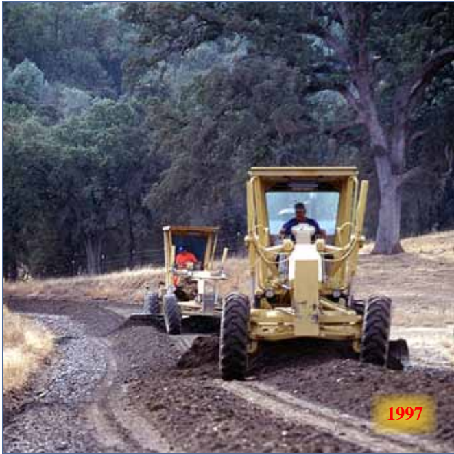
Following application of the liquid EMC SQUARED Stabilizer treatment to the asphalt millings and aggregate material, the treated aggregate mixture was processed by a tractor-drawn agricultural disk and motor graders, then shaped and compacted by vibratory smooth drum rollers.
