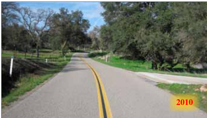
Asphalt pavement surface above stabilized base in excellent condition after thirteen years of service.
