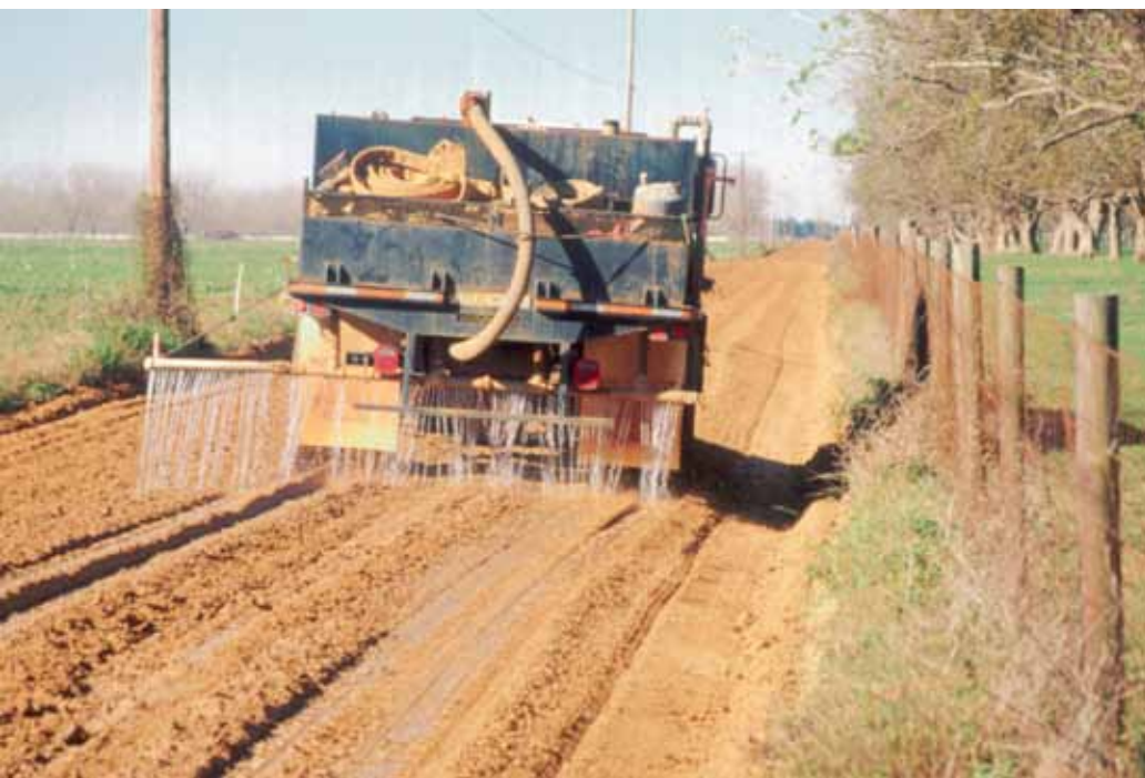
EMC SQUARED and EMS Dual Component Liquid Stabilizer products being applied in Baldwin County, Alabama.
