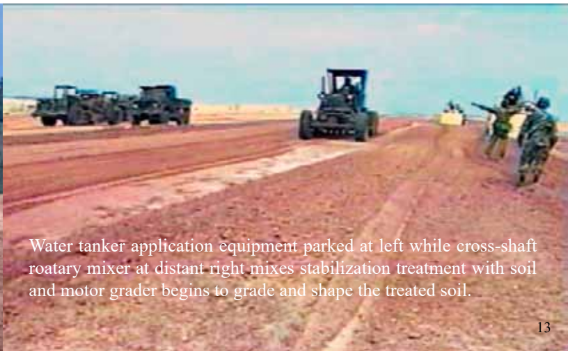
37th Engineer Battalion applying EMC SQUARED Stabilizer to Forward Landing Strip surface
