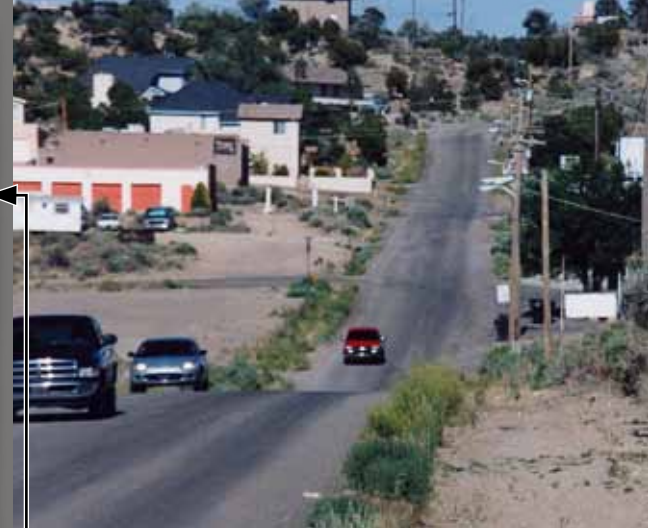
Asphalt Millings (RAP) Stabilized with EMC SQUARED Stabilizer (utilized for five years as a street surface)
